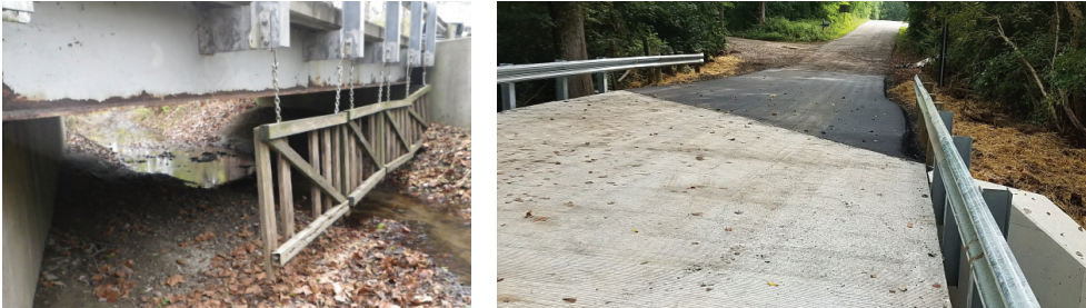
Left: Old steel beam/concrete deck bridge before replacement; Right: New Pence Jones Road Bridge #238-0.14
