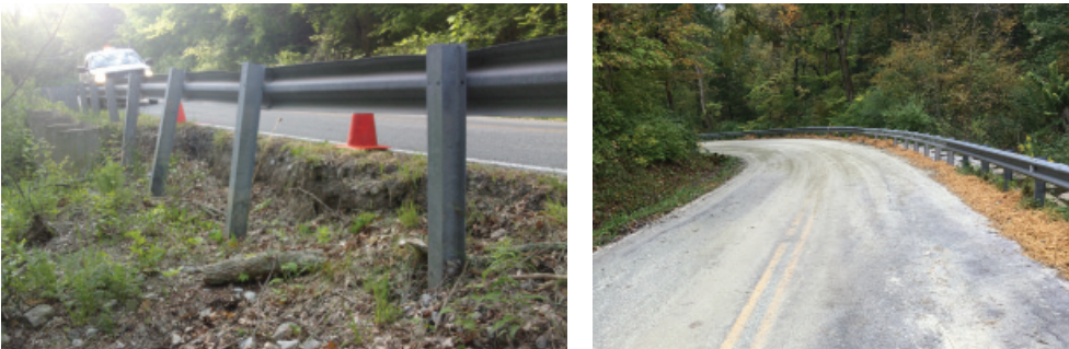
Left: road slippage on Olive Branch Road; Right: Completed roadway after construction of drilled pier wall
