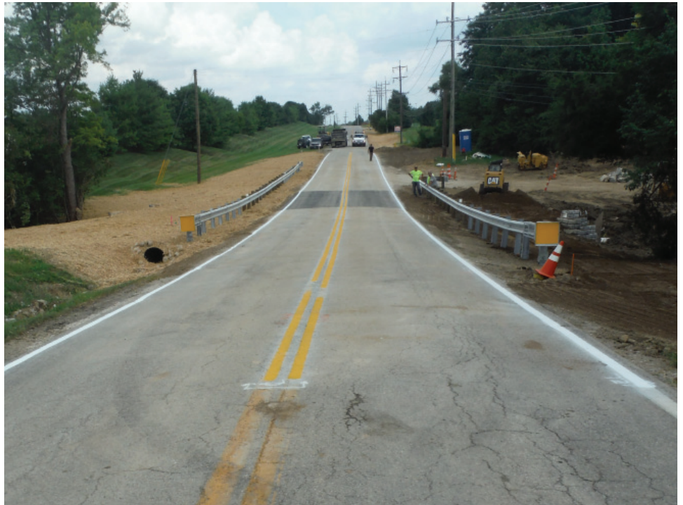
Above: Construction underway on Bethany Road Bridge; After: Completed Bridge Project on Bethany Road
