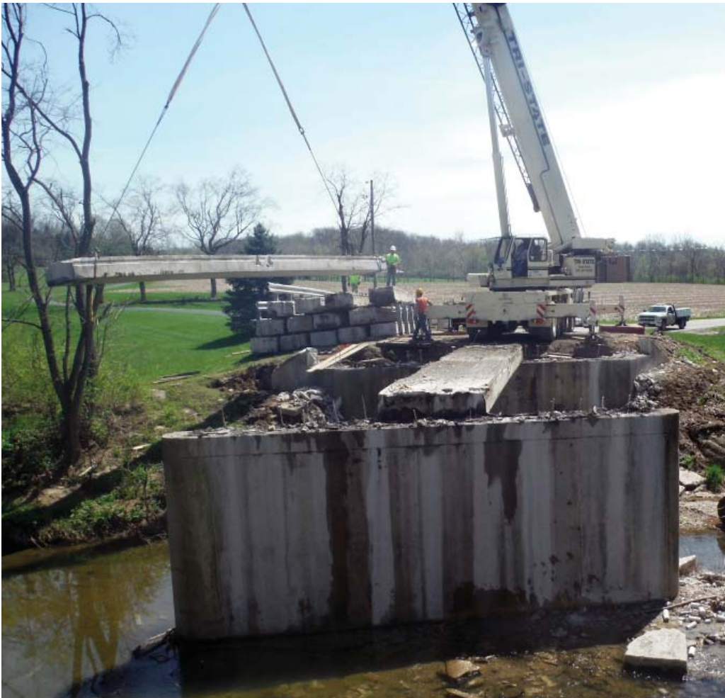
Old beams being removed from BR15-7.94 during rehabilitation project, completed this past summer.
