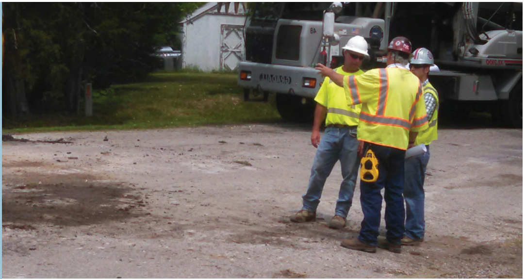
County Crew and Assistant County Engineer Dominic Brigano out in the field at BR195-0.11.
