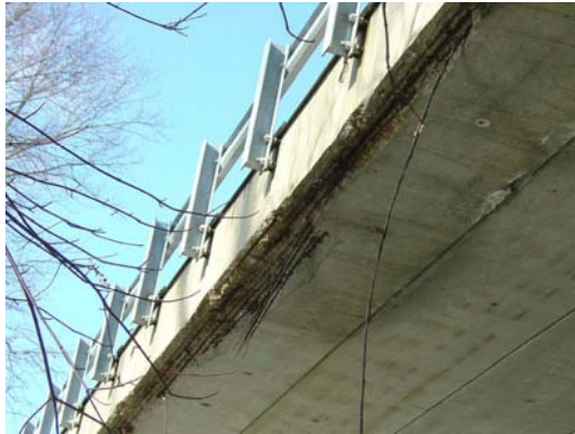
Wilmington Road bridge beam showing signs of deterioration.
